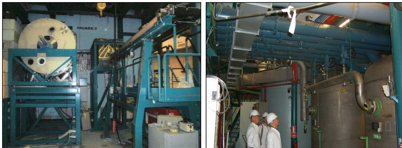
Figure 4. (left) DR 3, horizontal silicon facility; (right) secondary cooling systems.
